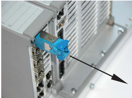
Figure 19: Deinstalling an SFP module
